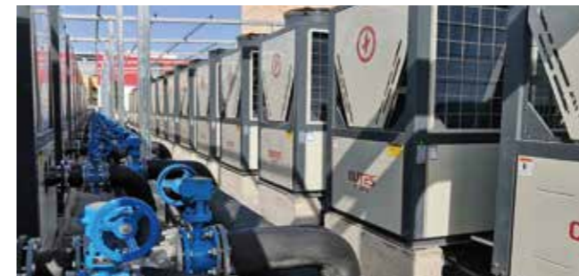
Liaoning Province Dalian City Vocational Technical School Heating Area: 150, 000m 2 Heat Pump: mixed models Total: 78Units
